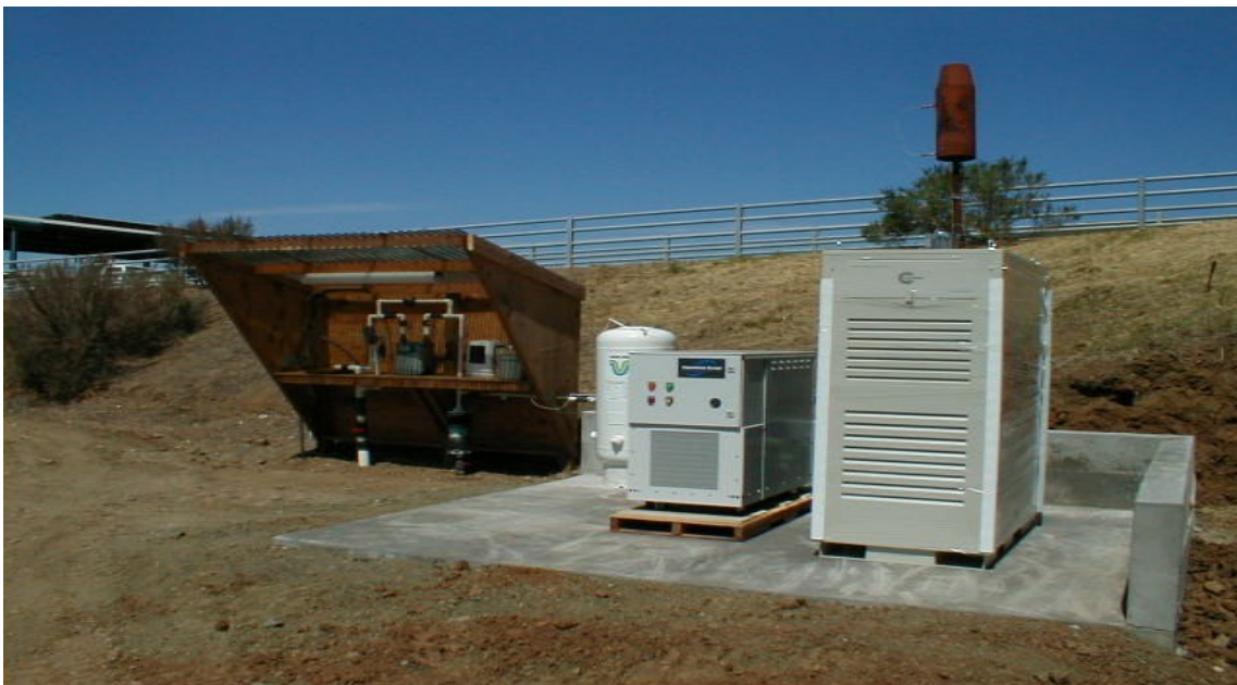
Figure 3: Biogas Handling System and 25 KW Microturbine Electric Generator
