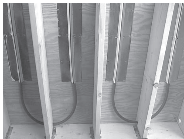
7/8" PEX in a floor Joist application
