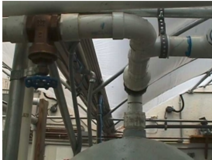
Picture 2 – Return water line from top of beadfilter to tank and hydroponic growing beds. Note bronze gate valve for cutting off flow to hydroponic unit.
