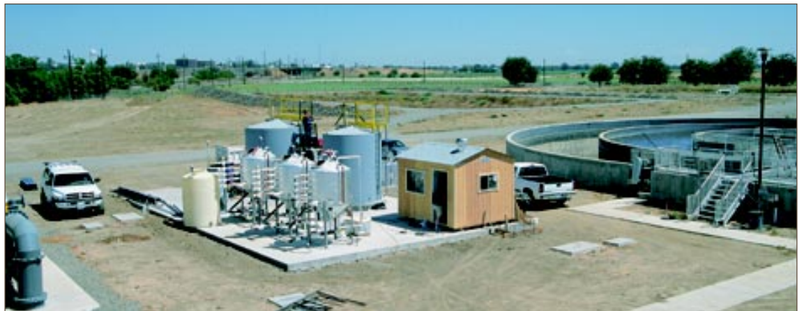
At UC Davis, a pilot plant is under construction of the APS-Digester, which converts animal manure and plant waste into biogas under anaerobic conditions. The first commercial application will be at a Florida racetrack, but it has broad applications for dairy, swine, poultry and other animal operations.
